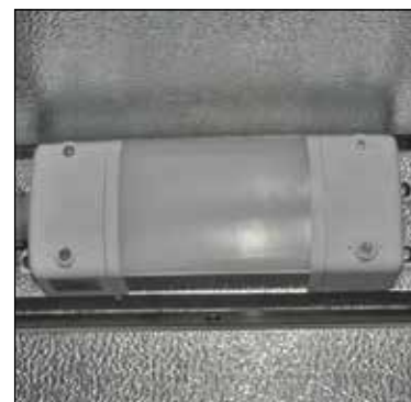
LED light fixture
